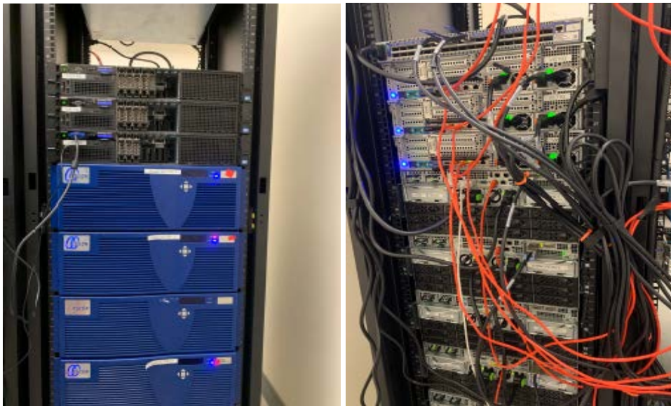
Figure 1. (Left) Front View and (Right) Rear View of Server Cabinet.
